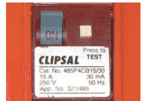
RCD's should be checked regularly
